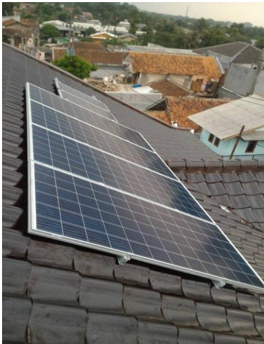
1.5 kWp Rooftop PV Off-Grid in Jakarta
