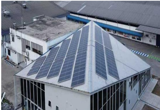
50 kWp Rooftop PV Hybrid on Textile Factory in Bandung
