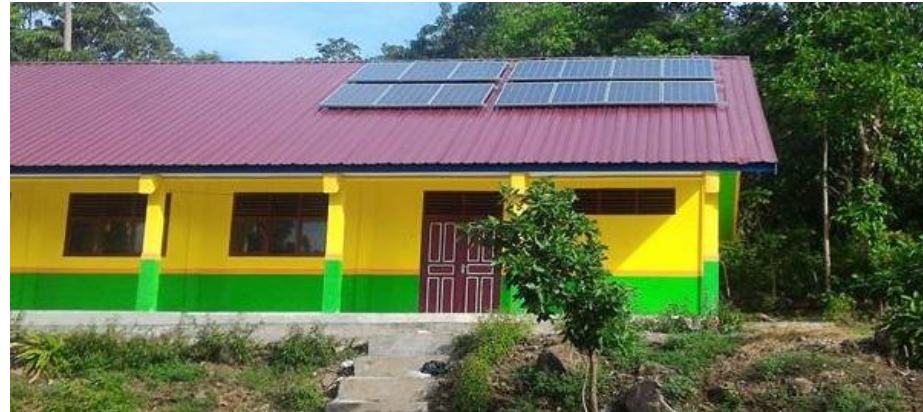
3.5 kWp PV with Hybrid inverter on school rooftop in Sulawesi
