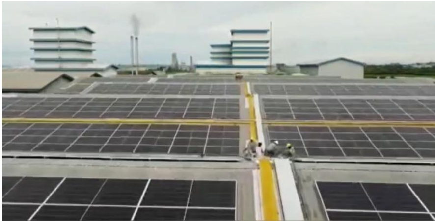
2 MWp PV Rooftop factory in Gresik
