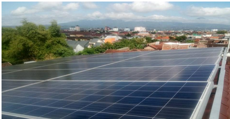
9 kWp Rooftop PV On-Grid in Surabaya
