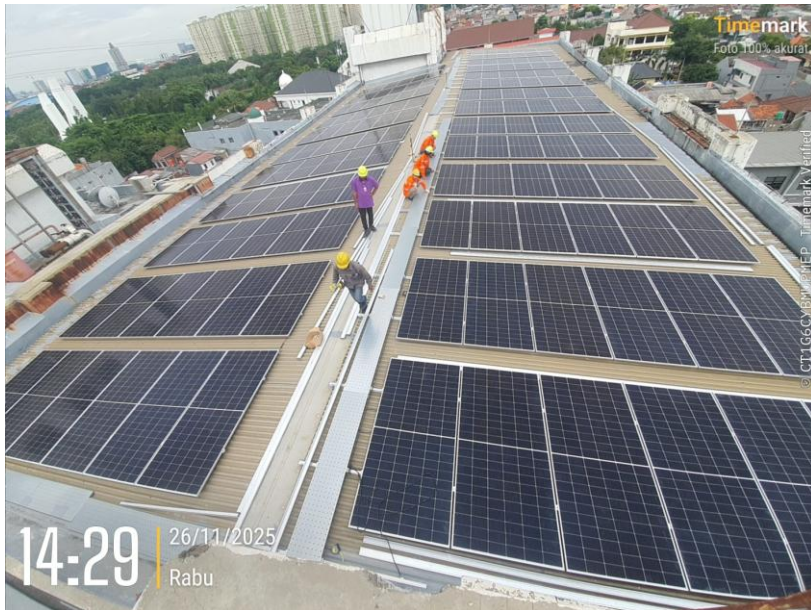
126 kWp PV Rooftop on PT Rekayasa Industri
