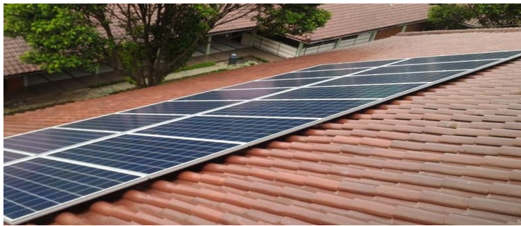
5 kWp Rooftop PV On-Grid in Depok
