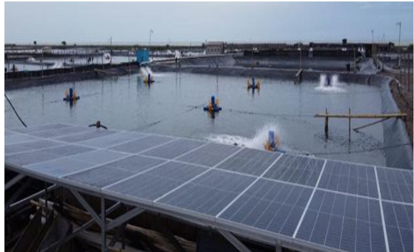
20 kWp PV Ground Mounted in Shrimp Farm
