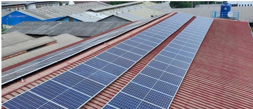
40 kWp PV Rooftop F&B factory in Jakarta
