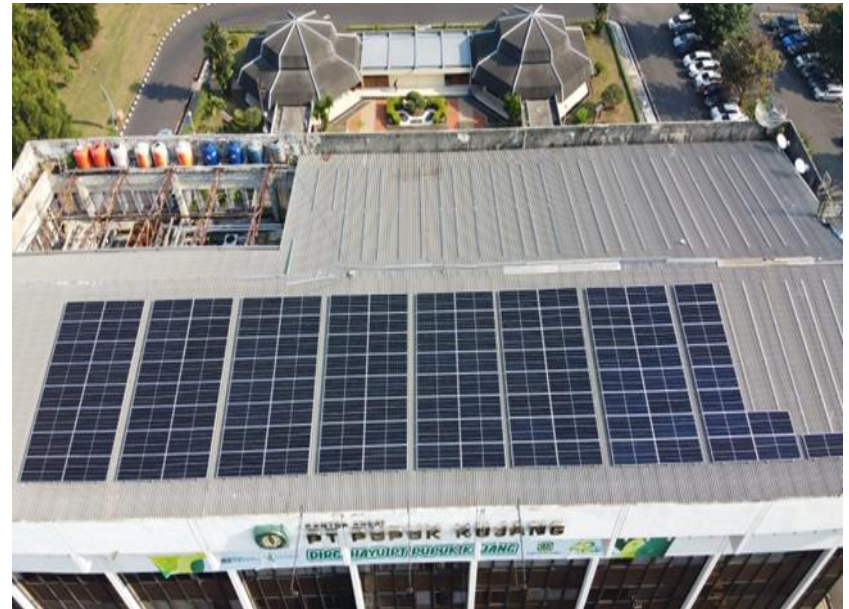
133 kWp PV Rooftop on PT Pupuk Kujang
