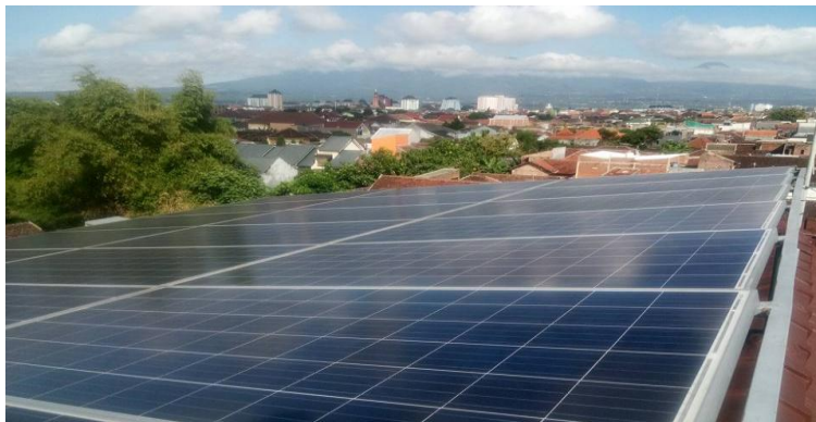
9 kWp Rooftop PV On-Grid in Surabaya
