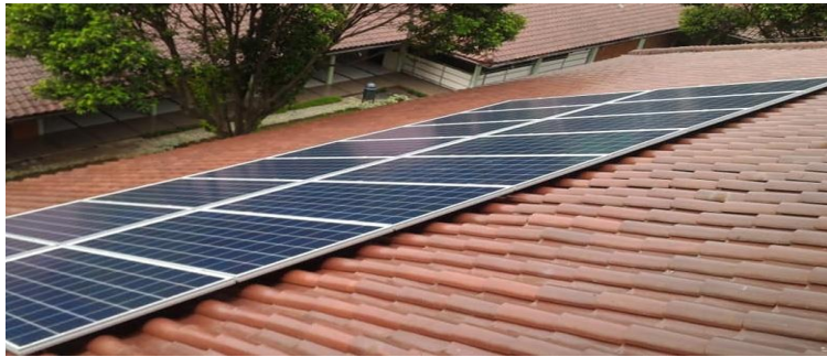
5 kWp Rooftop PV On-Grid in Depok
